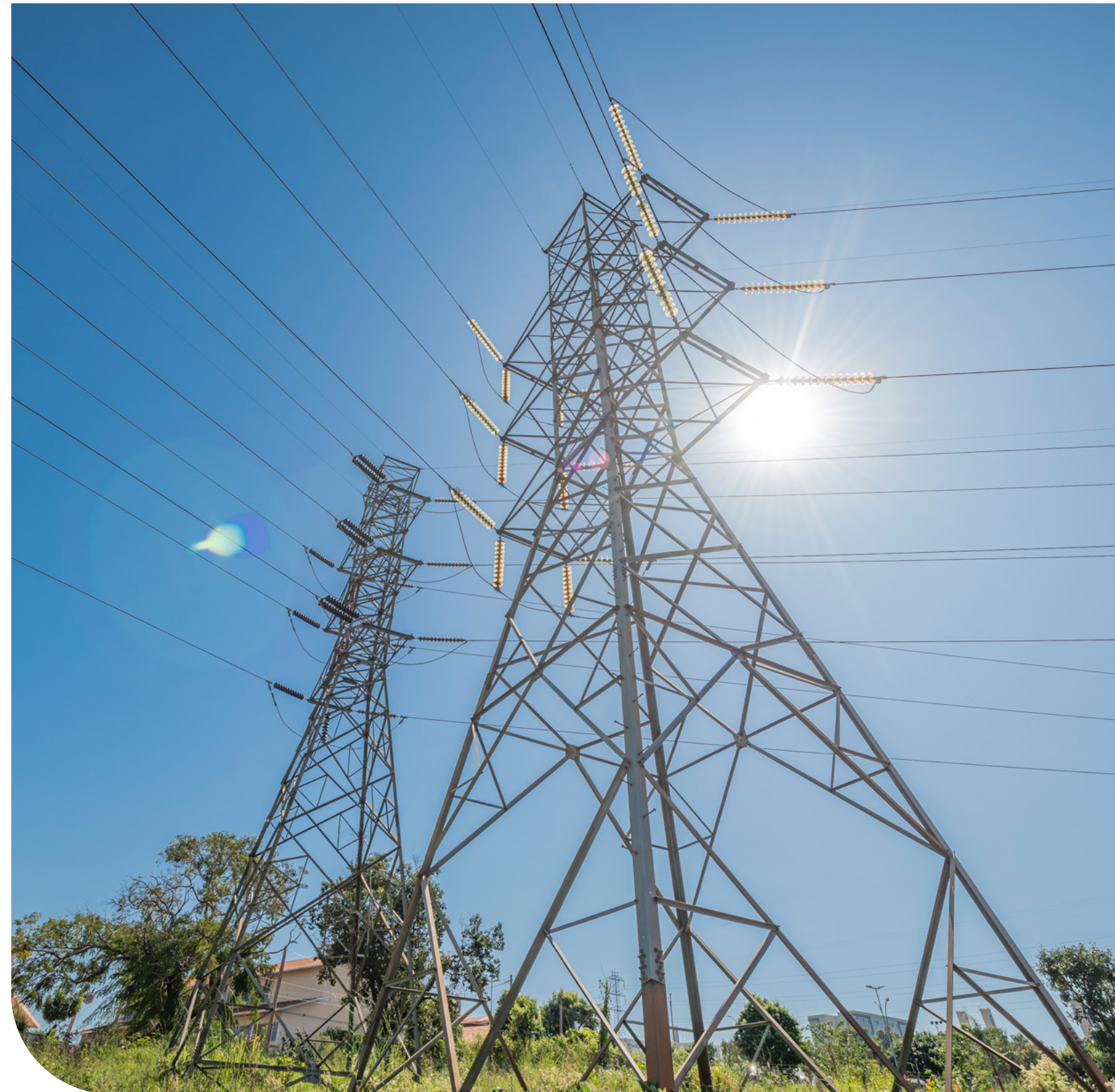
Sub-transmission towers in Araraquara (SP).
