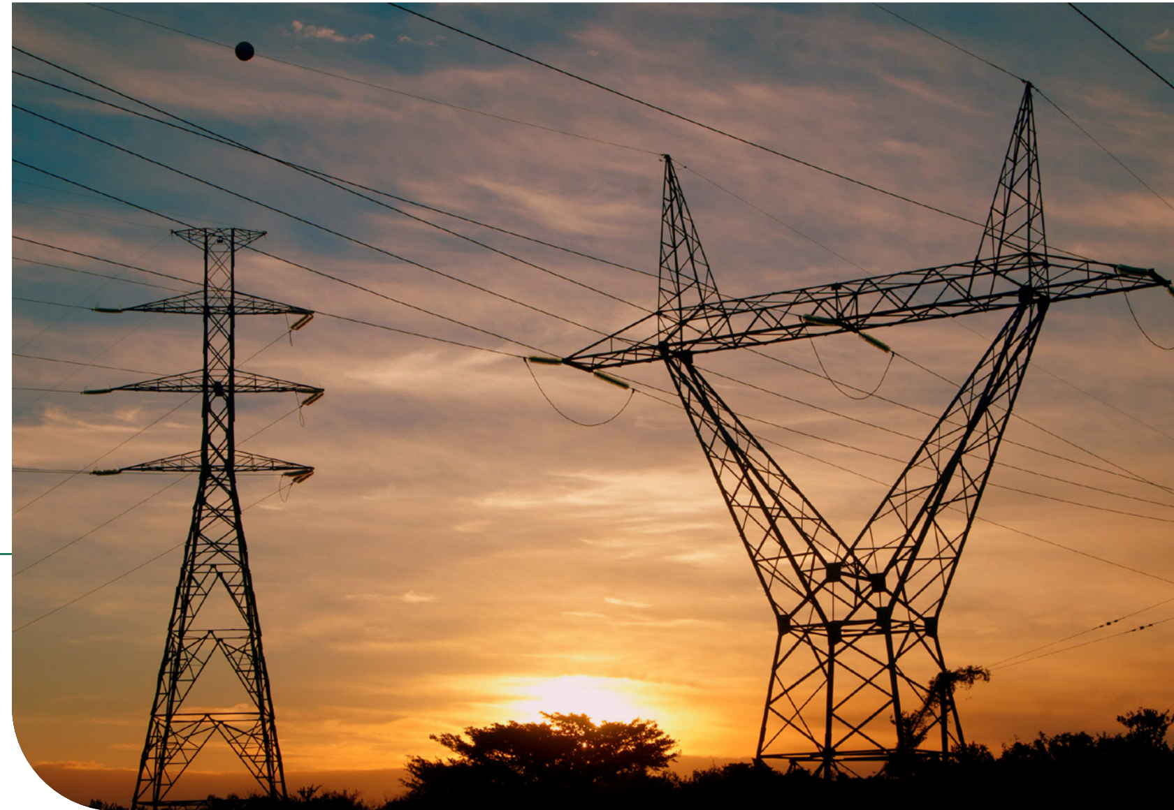
Transmission line in Rio Grande (RS).
