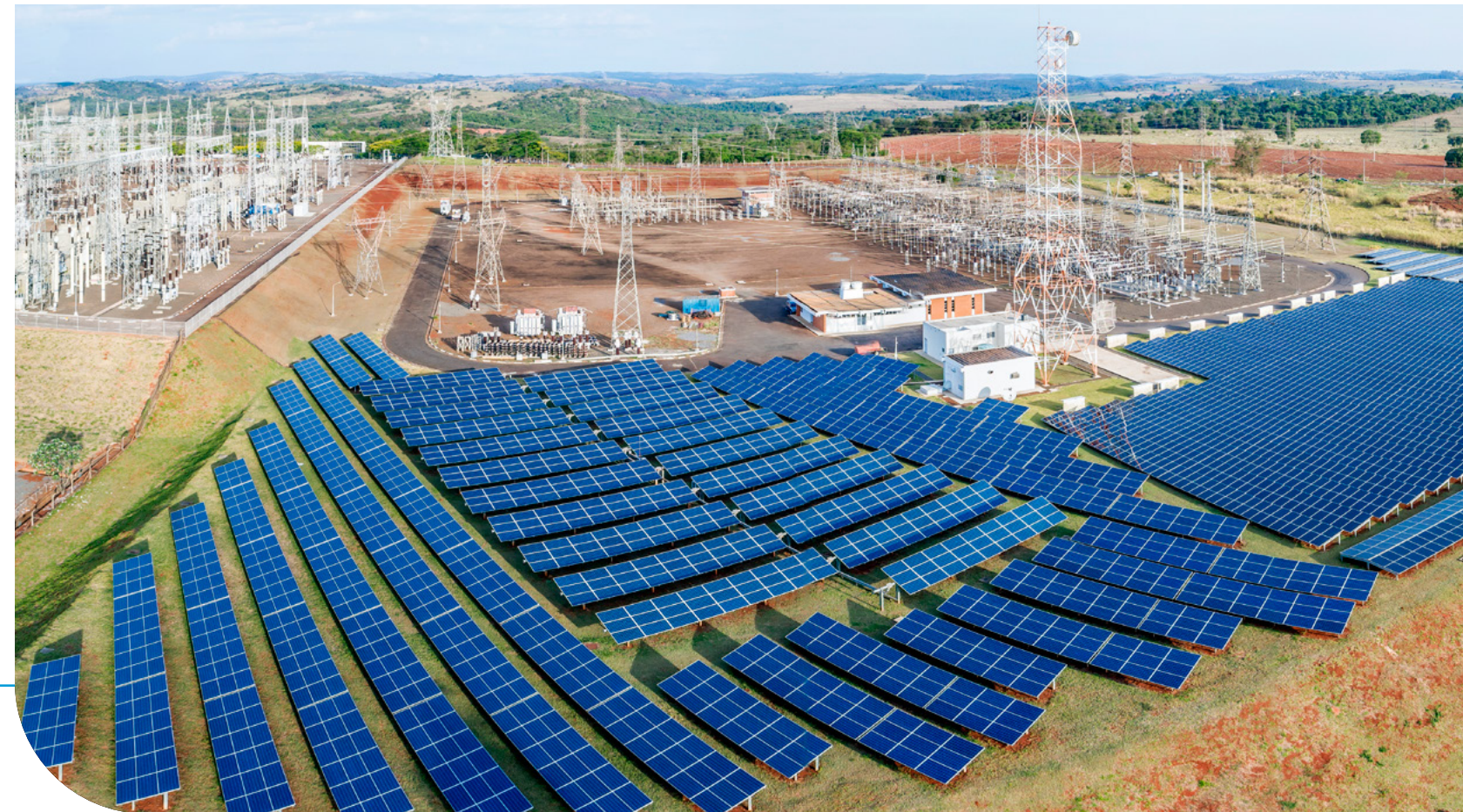
Tanquinho Solar Power Plant, in Campinas (SP).
